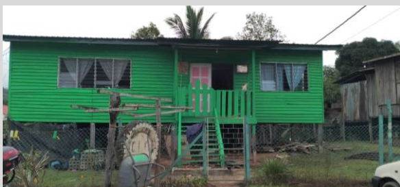
The school building underwent a few renovations such as a repaint, new back staircase and ceiling board replacements.
